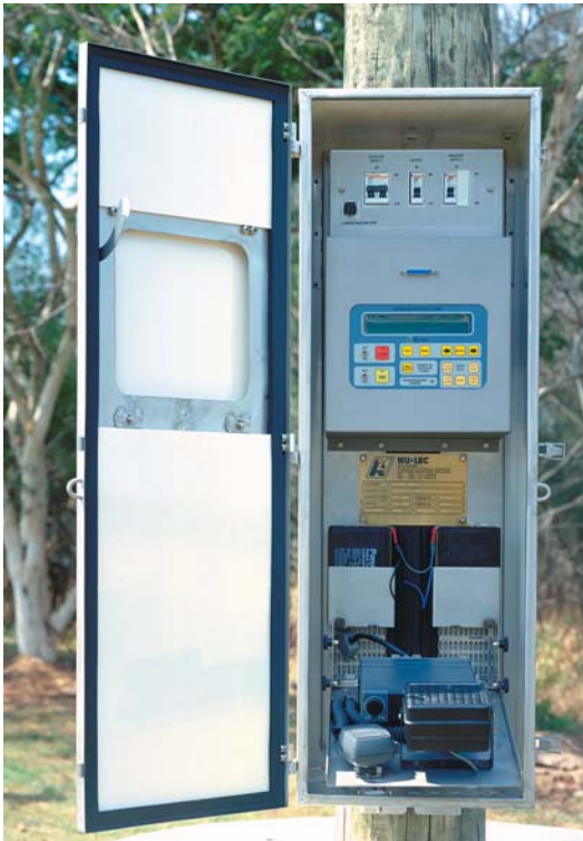
Pole Top Control & Communications Cubicle
